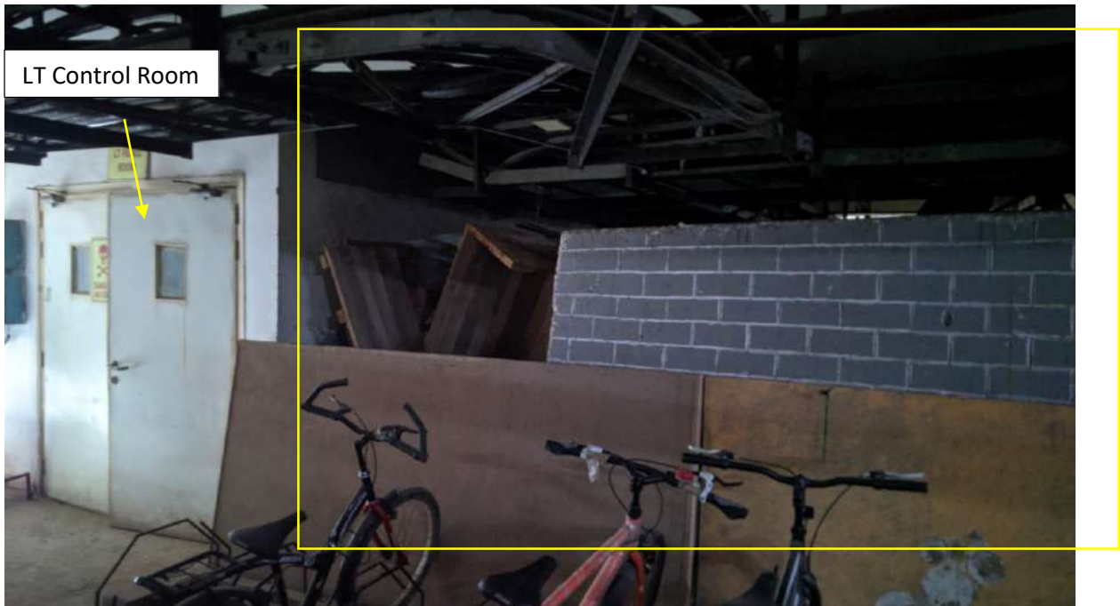
Side view of space for BESS installation, Entry to LT Control Room, cable trays, debris present
