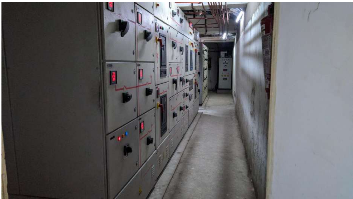
Inside view of LT Control Room
