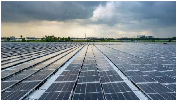
Photo 2: The 60MWp Sembcorp Tengeh Floating Solar Farm
