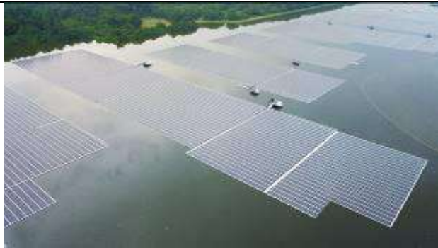
Photo 1b: Aerial view of the Sembcorp Tengeh Floating Solar Farm
