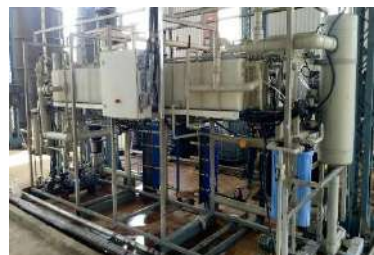
Acid Recovery Plant
