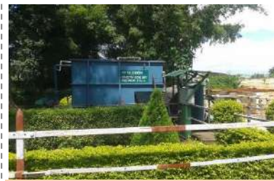
STP plant for waste water treatment
