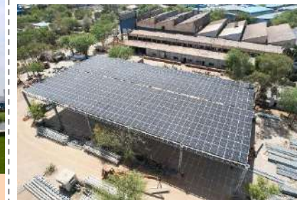
Solar rooftop plant
